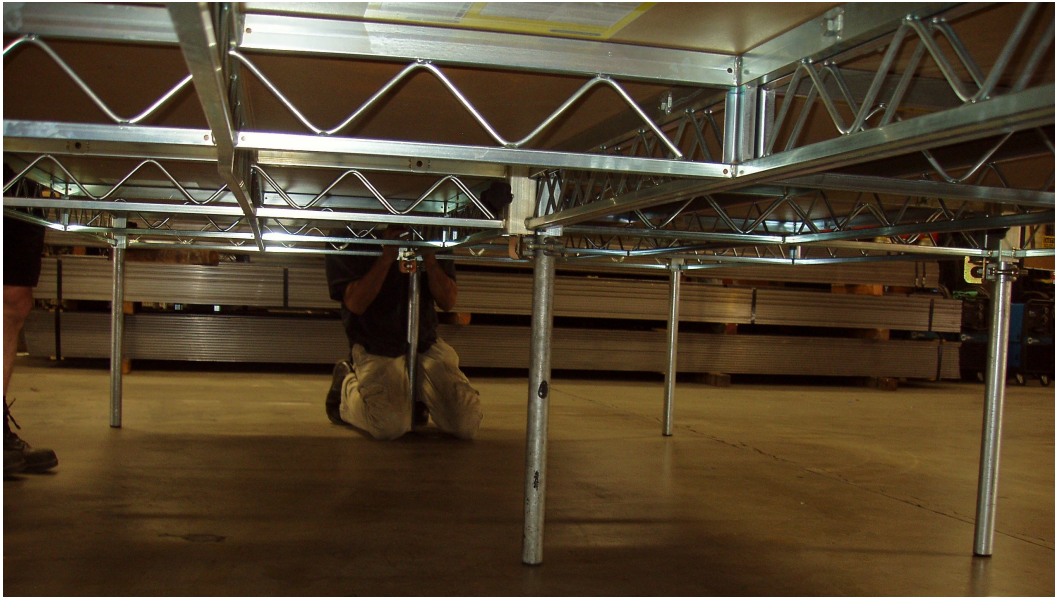
Figure 2-2 Test Platform, View from below of Critical Central Leg
