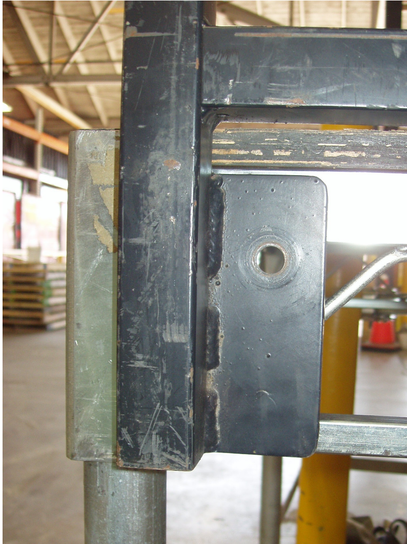
Figure 3-9 Guardrail bottom joint after tests #1-3
