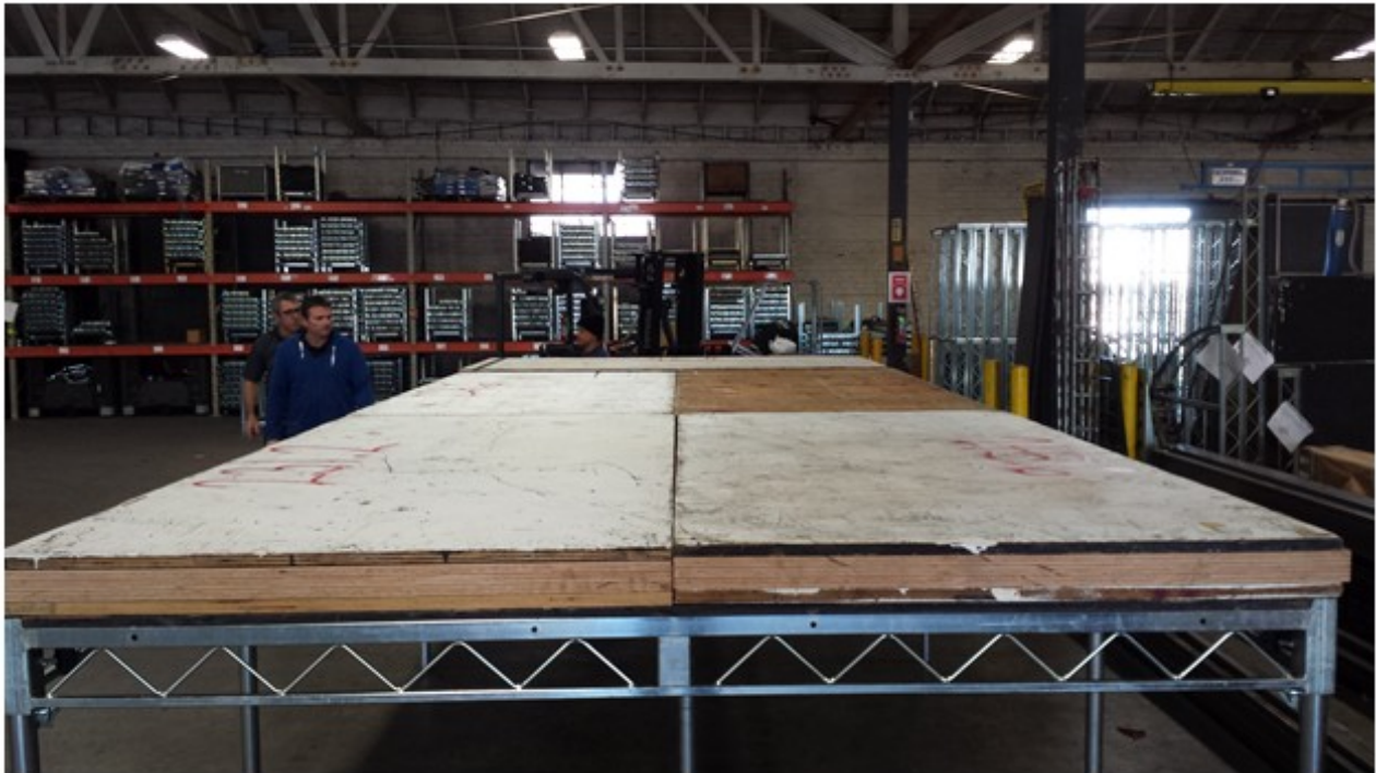
Figure 2-8 4 ft. tall 8x20 ft. Platform with wooden pallets in place, overlapping deck seams
